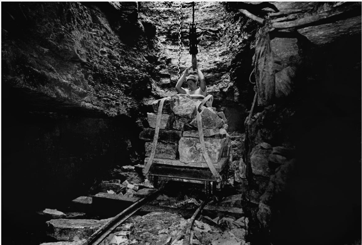
At the foot of the vertical shaft the crane hook is about to be attached to the slings which are attached at the corners of the flatbed cart. 1982.
